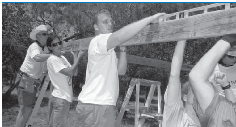
Volunteers of the First United Methodist Church of Edna work together to renovate an outdoor chapel at Methodist Mission Home.
